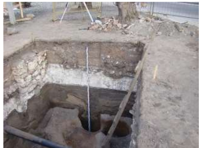
Fig. 4. Tver. Dug-pit made in 2011 in the south-eastern corner of the cathedral garden.
