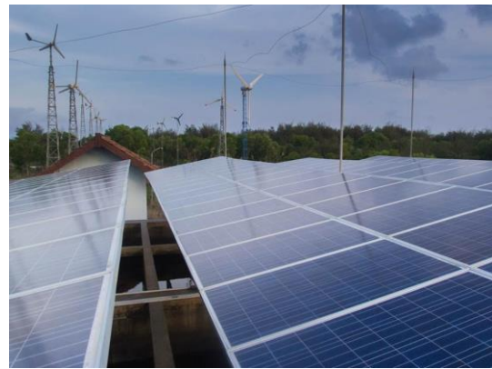
Figure 1. Hybrid Power Plant in Pantai Baru
