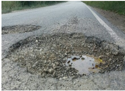
Fig. 3. Road damage in Meredan, Siak, Indonesia, 2015.
