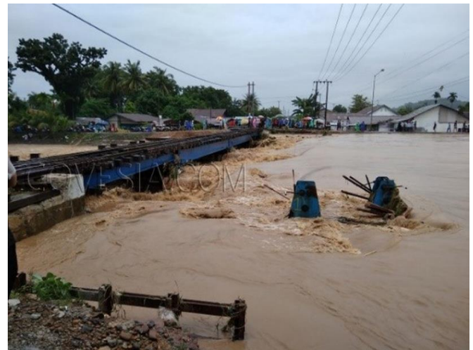
Fig. 1. The railroad bridge is almost flooded.
