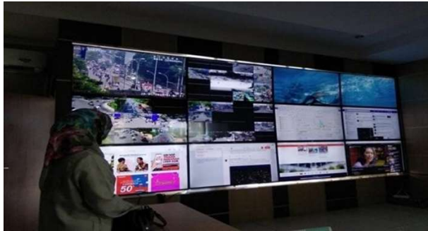
Fig. 10. Central control unit mounted on DISHUB Semarang.
