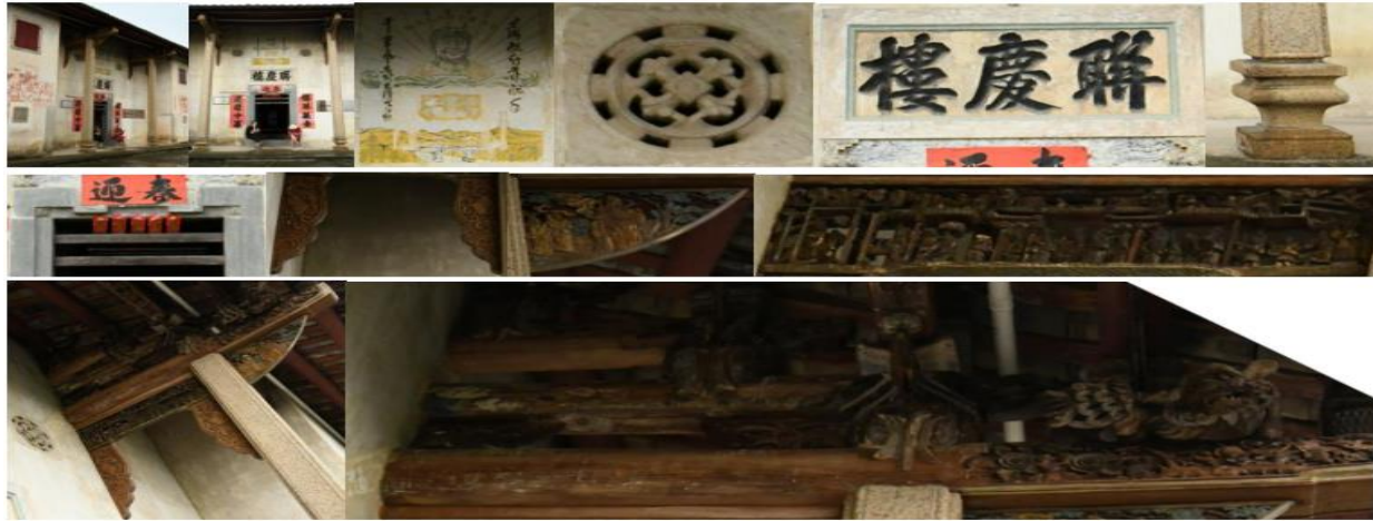
Fig. 4. Decoration of the facade of the concave belly gate; "Depending on Mao Zedong Thought to Carry out the Revolution, Depending on the Helmsman to Sail on the Sea" propaganda poster of Chairman Mao during the Cultural Revolution; Ruyi line ventilate stone windows on the second floor; stone plaques on the building name; four-sided beamed stone pillar foundations, gate hairpin, outrigger, sparrow brace, hollow sculpture of lion.
