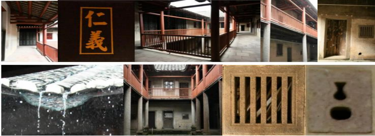
Fig. 5. Beam-lifted bucket arch on the second floor; gold characters plaques; columns, beams, and railings of different cylindrical combinations of vermilion formed around the courtyard; under the corridor on the second floor are purlins and beams to support; ordinary stone door frames in the courtyard and stone mullion windows; weak mixing angle gutter tiles at the four corners of the courtyard; mullion windows; straight railings and handrails; gourd-shaped gun squint for defense.
