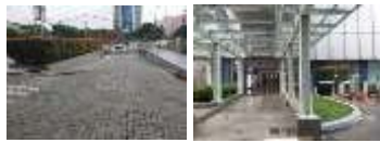
Figure 12: Damaged Pedestrian paths.
