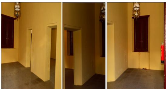
Figure 11 The inner wall of the ammunition warehouse
