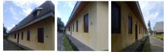
Figure 12 The inner wall of the ammunition warehouse
