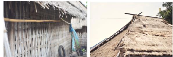
Figure 11 Woven bamboo panel as wall material, and dried reed grass as roof
