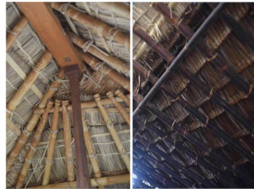
Figure 10 Kecapi wood as roof easel frame, and bamboo as roof rafter frame
