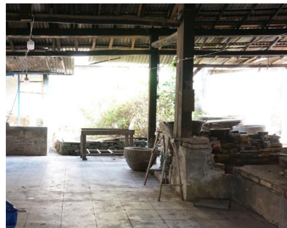
Figure 8 The well at the open area of the kitchen and the stove at few meters to the north. (H. Rani, 2019)
