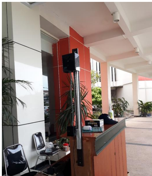
Figure 7 Complete view of temperature detection system
