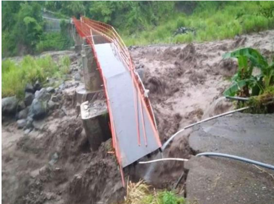
Figure 1 The collapse of the Plompong Bridge, Brebes Source: Sucipto I.(2019).
