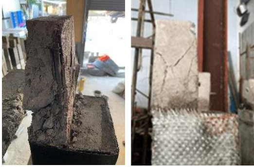
Fig. 5. Failure of strengthened columns using CFRP laminates (left) and GFRP laminates (right).
