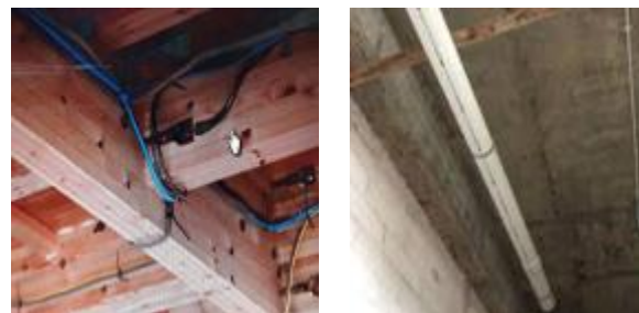
a. Electrical installations b. Sewerage installations
