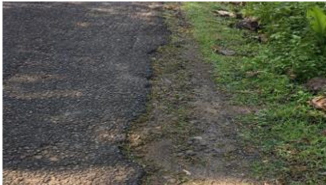
Fig. 7. Edge cracking at the location
