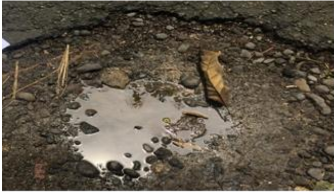
Fig. 6 Potholes at the location
