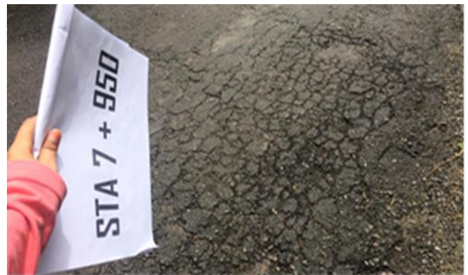
Fig. 4 Alligator Cracking at the location STA 7+950
