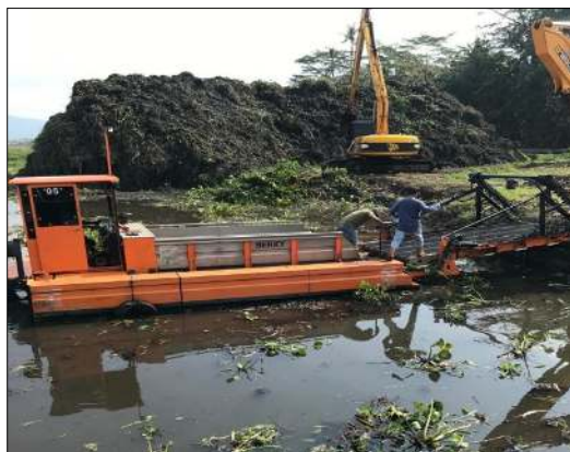
Figure 2 Heavy equipment to transport water hyacinth to the edge of the swamp
