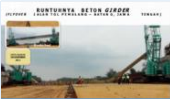
Fig. 3. The collapse of Girder concrete
