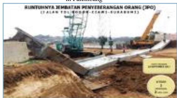
Fig. 2. The collapse of the People Crossing Bridge, In September the collapse of the People Crossing Bridge (JPO) on the Bogor-Ciawi-Sukabumi Toll Road the collapse of the pedestrian bridge on the Bocimi toll road,
