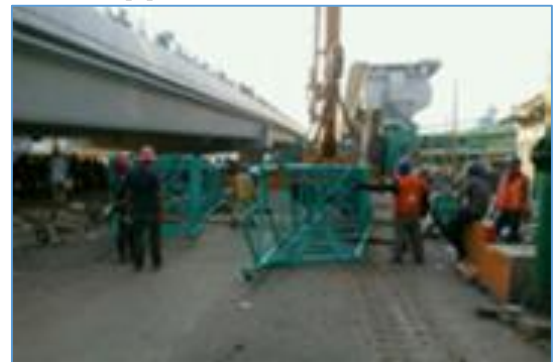
Fig. 1. The fall of the crane The fall of the crane in Palembang, Major Construction Accidents: In August the fall of Crane (Light Rail Transit) in Palembang
