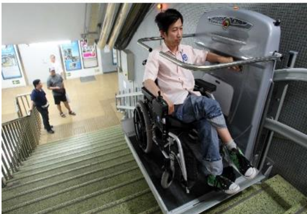
Figure 12 Stairway lift in Chegongzhuang, Beijing Metro Source: http://www.china.org.cn , accessed on May 10 th , 2019
