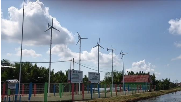
Figure 1. EMAS BAYU Hybrid Power Plant in Bondan hamlet, Cilacap, Indonesia
