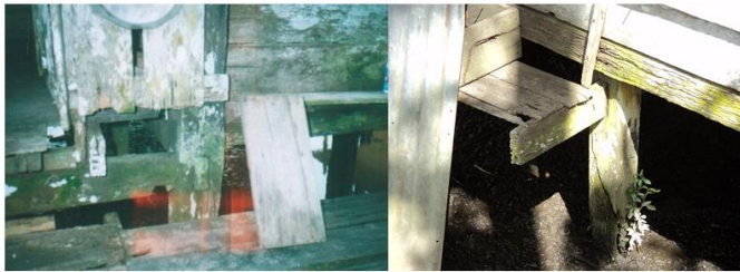
Fig. 3. The mildew attacks the floor joint of West Kalimantan's traditional house (the picture taken of the houses in Sambas Town).
