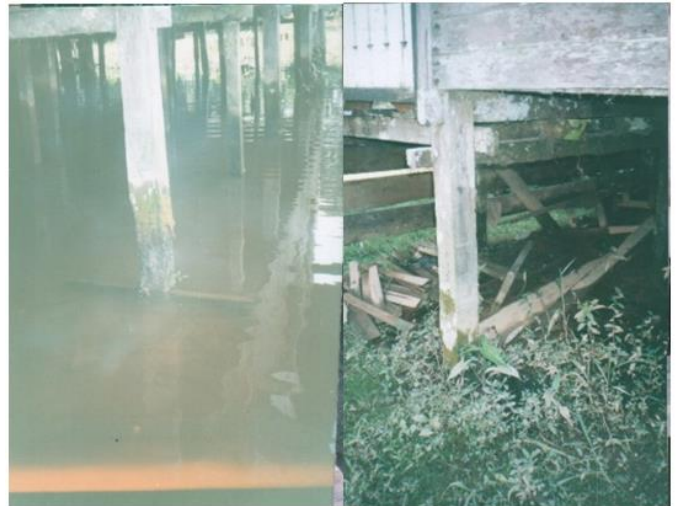
Fig. 1. The condition of wet-dry to the foundation of West Kalimantan's traditional house (the picture taken to the houses in Sambas Town).
