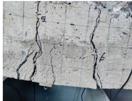
(b) The crack pattern in Specimen AN
