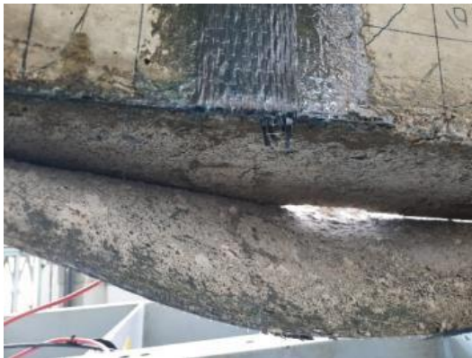
(b) Broken of CFRP U-Wrap
