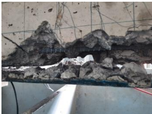
(c) Concrete Cover Separation
