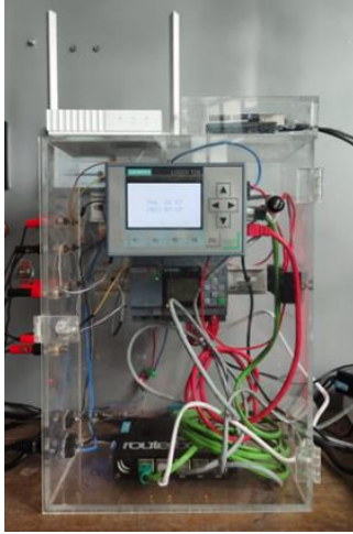
Figure 9 Remote accessible box
