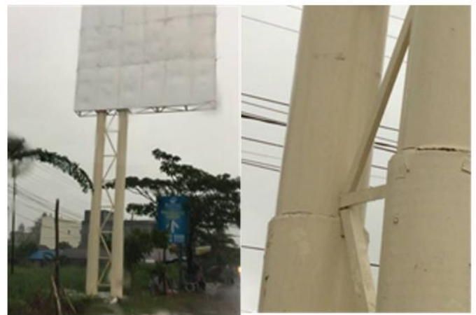
Fig. 1. The failure on the billboard pile connection.
