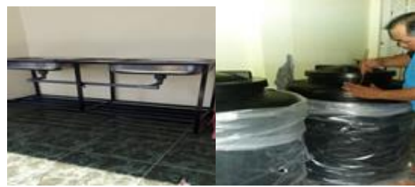
Figure 2 Mini WWTP design at UKM Batik Sidomulyo (top left) Place for batik dyeing and coloring process (top right) Tank for mixing and purifying batik wastewater with bacteria media and plastic ball (bottom) pump for power in the stirring process
