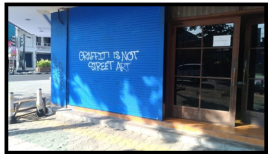
Figure 5. Vandalism in Gatsu. Source: Apika, 2020
