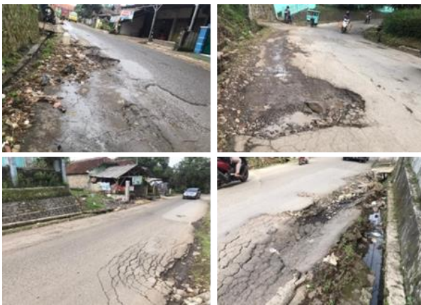
Figure 3. Pavement distresses in Cikalong-Cipeundeuy road.
