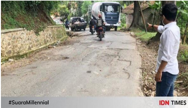
Figure 2. Damaged road due to heavy loading KCIC Project (IDN Times Jabar, 2021).
