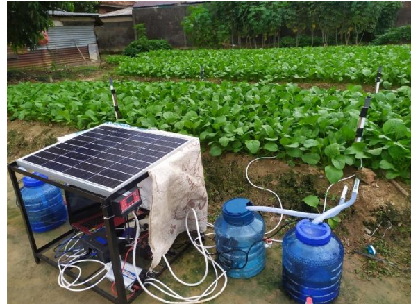
Figure 3 Testbed of the solar powered automatic sprinkler system
