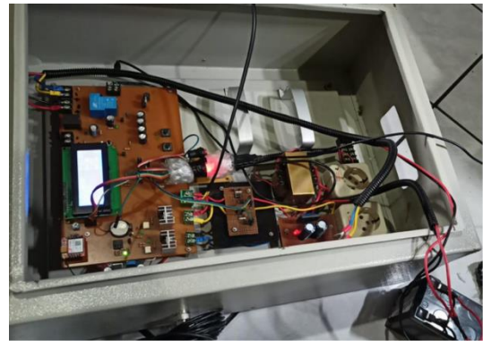
Fig. 3. Circuit box controller.
