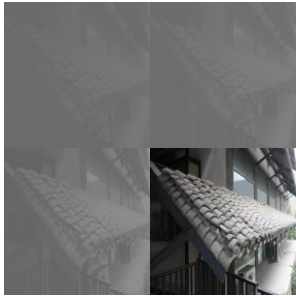
Figure 3. Increased brightness of eave tiles in wooden buildings
