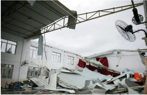
Fig. 1. The impact of Typhoon Rammasun on houses in Haikou city
