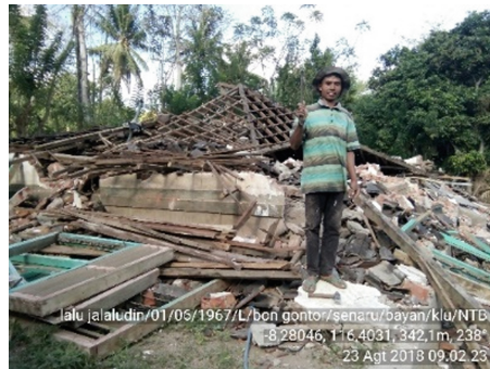
Fig. 4. Photo of House Damage due to Lombok Earthquake 2018
