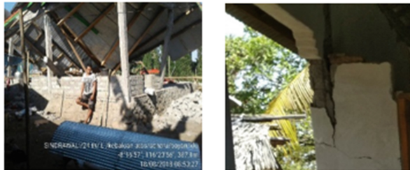
Fig. 12. Damage to Columns and Column-Beam Connections in House Buildings
