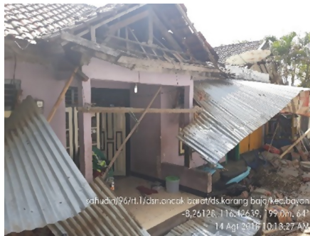
Fig. 16. Roof damage due to the absence of reinforcement/stiffening between the walls or beams with the roof
