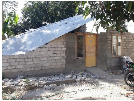
Fig. 5. No foundation and sloof structure in the building
