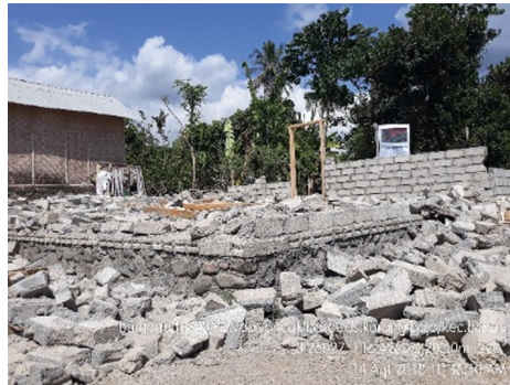
Fig. 6. Sloof Structure is not present in Building
