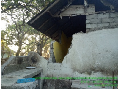
Fig. 11. Building Houses without Reinforcement of Columns and Beams
