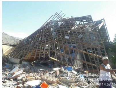
Fig. 10. Wall Damage Category Heavy Damage
