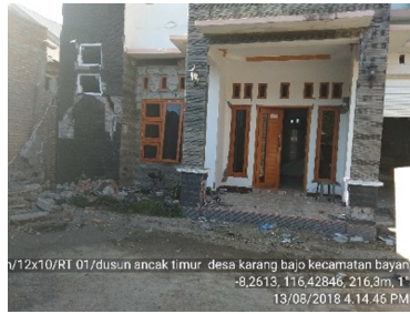
Fig. 9. Damage to the wall in the category of moderate damage
