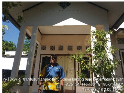
Fig. 8. Damage to the wall in the category of light damage
