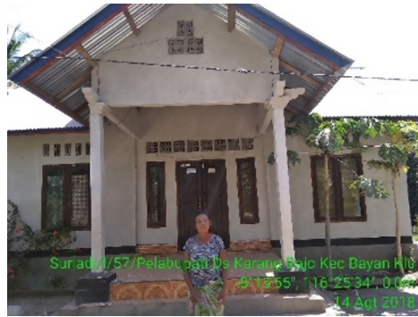
Fig. 7. Typical Damage to buildings with sloof and foundation structures
