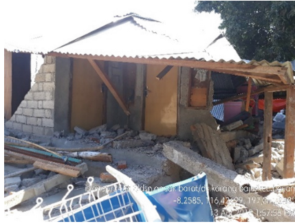
Fig. 15. Roof damage due to collapsing supporting walls
