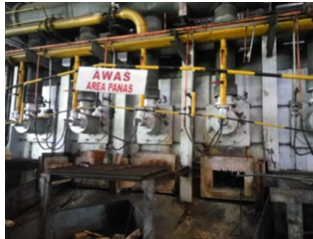
Fig. 7. Burner. Source: Personal Documentation
