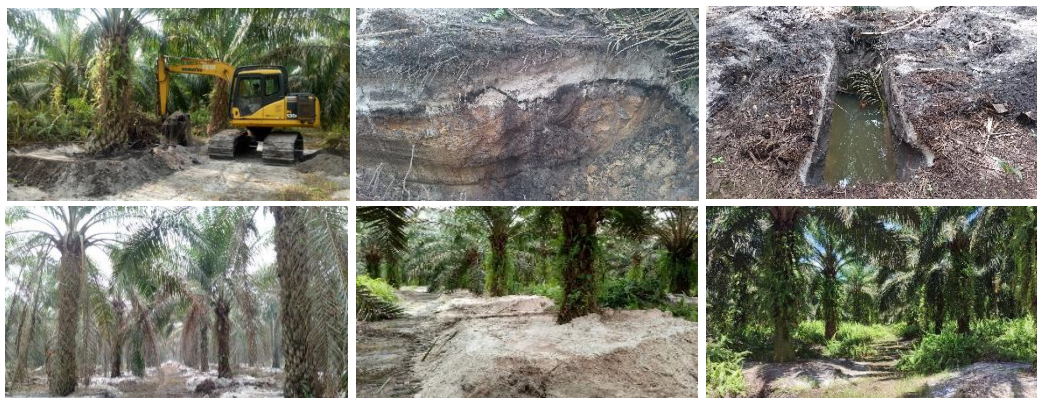
Figure 1. Application of hardpan breaking and mounding on spodosols in oil palm plantation
