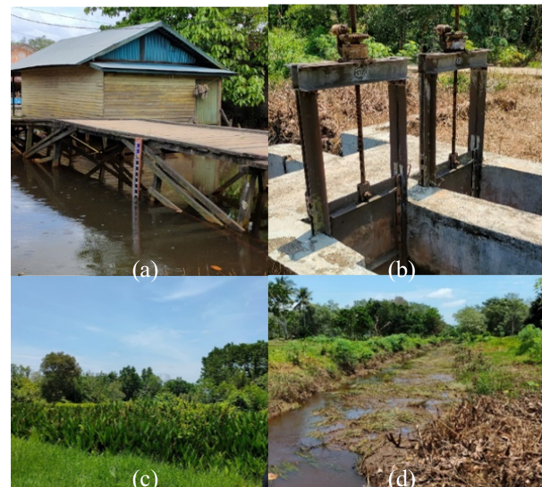
Figure 6 Existing Condition of the Unit Tamban such as (a) settlements around the primary canal, (b) damaged water buildings, (c) settling pond full of shrubs, and (d) sedimentation of the canals
