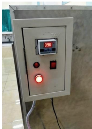
Fig. 5. Box Control Cabinet Dryer Based Automation
