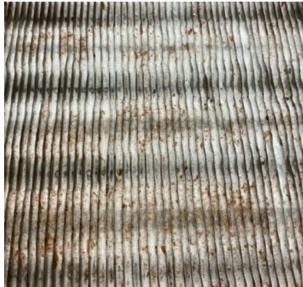
Fig. 3. Solidified organic salt in the fin-tube heat exchanger of the PCM storage.
