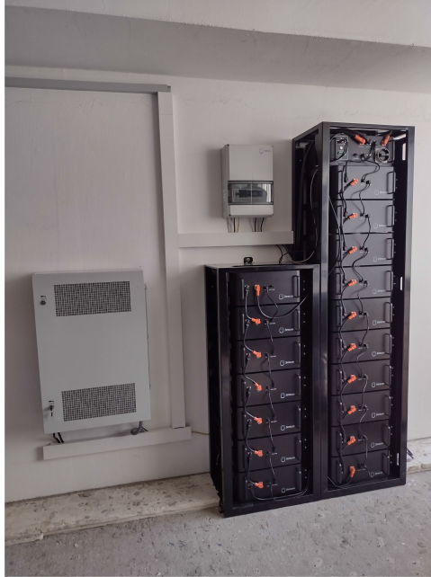
Fig. 4. Lithium Iron Phosphate technology based ESS installed at student residence (Image courtesy: Stage76 Administration)
