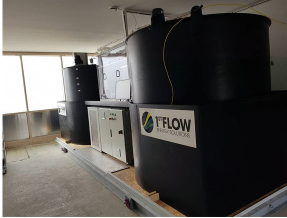
Fig. 3. Vanadium Redox Flow Battery installed at student residence. (Image courtesy: 1st Flow Energy Solutions GmbH)
