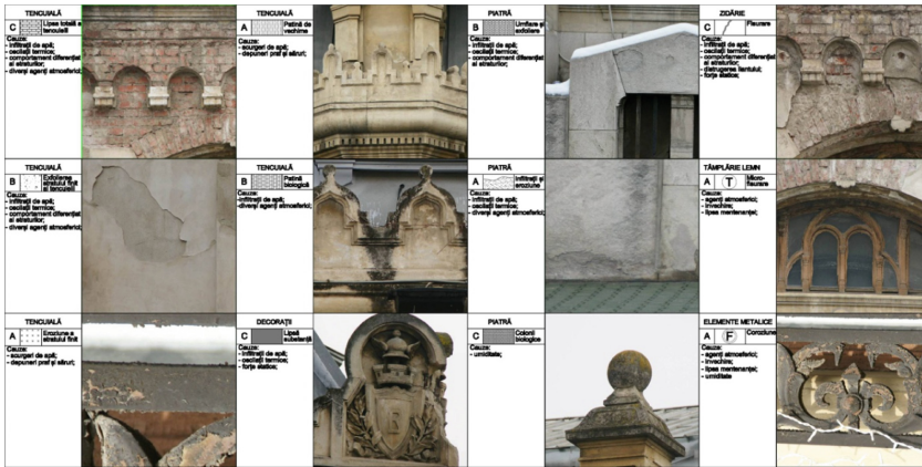
Fig. 5. The facades degradations investigation. Project by Getrix S.A., Craiova
