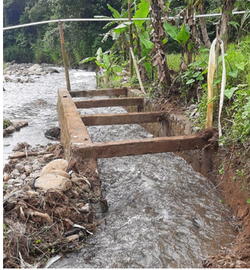
Fig. 1. Waterway and concrete construction in which small hydro power generation unit is installed.
