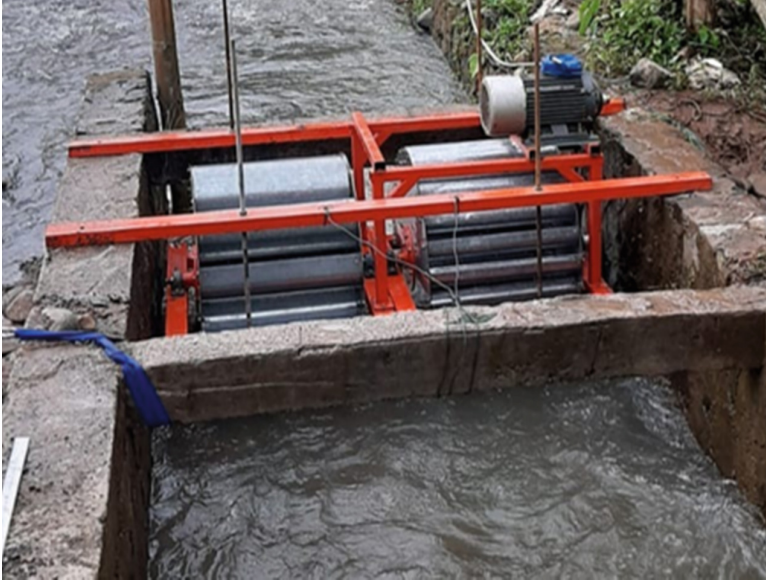
Fig. 4. The small hydro power generation unit installed in the waterway.
