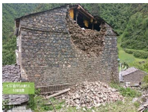
(c) 脚木足乡蒲市口村石木结构墙体局部垮塌
