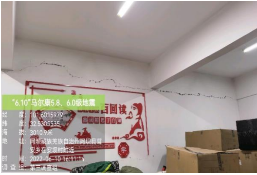
(a) 茸安乡安坝村框架结构墙体裂缝
