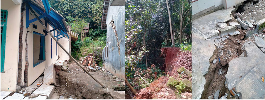
Fig. 1. Land subsidence in Curugpanjang
