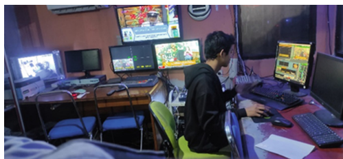
Fig. 2. Control room. (Photo: Budi/ Dhoho TV)
