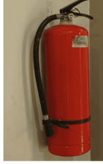
Fig. 5. Light fire extinguisher.
