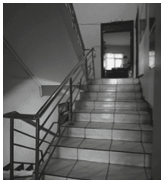
Fig. 4. Stairs that already use stair railings.
