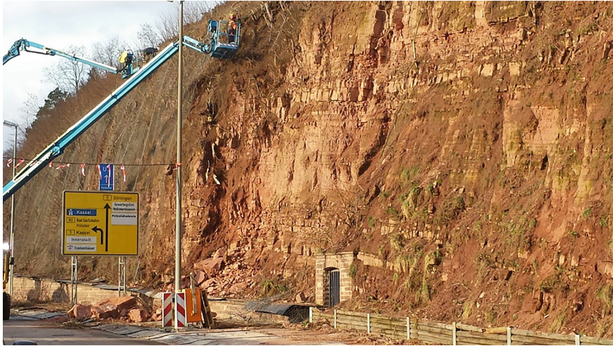
Fig. 2. Rock face in sandstone with strong signs of alteration after about 55 years of standing.
