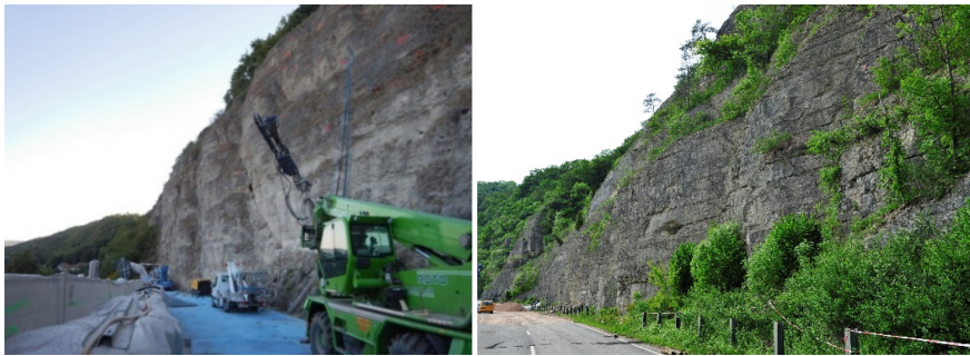
Fig. 5. Two construction projects (Dornburg-Camburg and Holzminden) which are geologically very similar but 200 km away from each other
