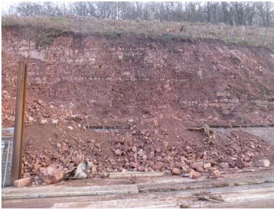
Fig. 6. Sandstone slope with the eroded weathered layer.
