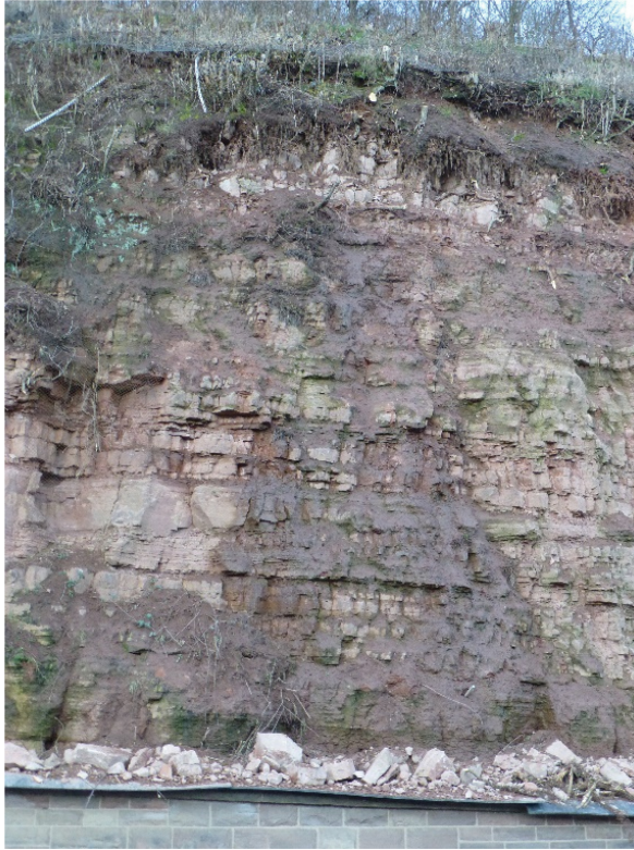
Fig. 8. Fissure water leakage (intermittently, after precipitation) from the sandstone slope
