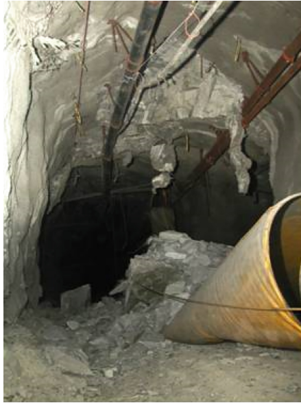
Fig. 8: Damage from a \sim 1.5 M_L near field event – note that FOG largely between support elements
