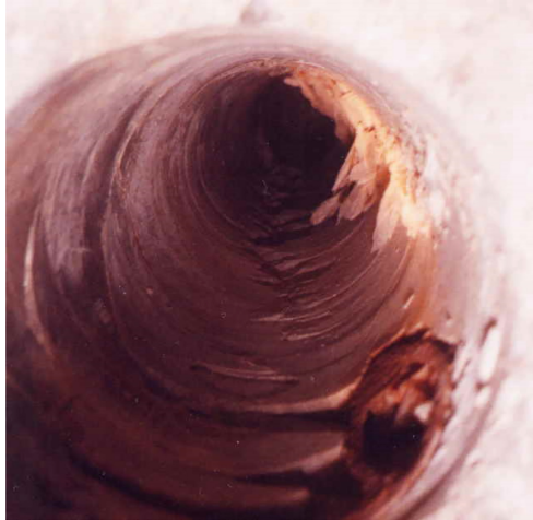
Fig. 4: Brittle spall of a bore hole wall
