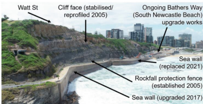
Fig. 1. Looking north to South Newcastle Beach, showing overall site setting, sub-vertical cliff face, current rockfall protection fence, Bathers Way coastal walkway, sea walls and recent works (photo taken on the 16/12/2022)
