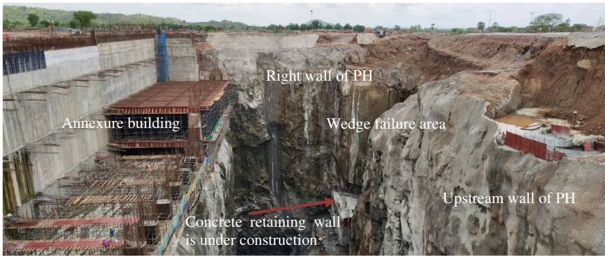
Fig. 4. View of wedge failure and concrete retaining wall is under construction
