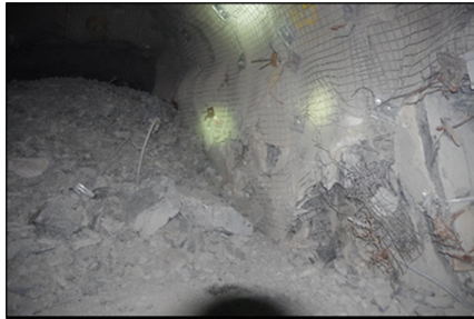
Fig. 3. Buckling in sidewalls due to combination of stress and foliation.
