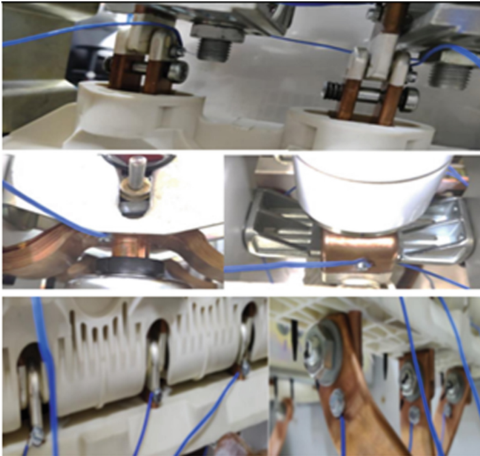
Fig. 2. Thermocouples at crucial spots in Switchgear assembly (Courtesy: M/s.ABB India Ltd.)
