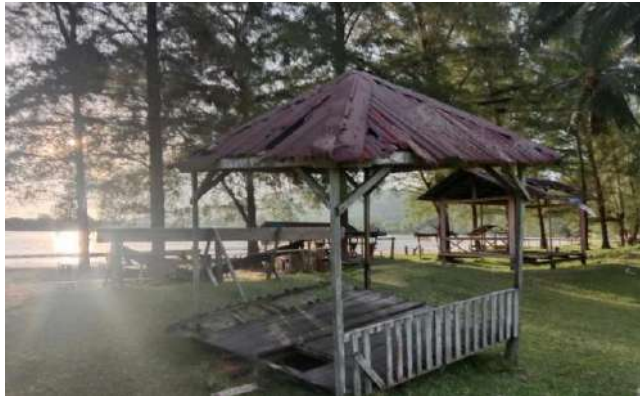
Fig. 3. Damaged facilities on the edge of the busung beach (Research documentation)
